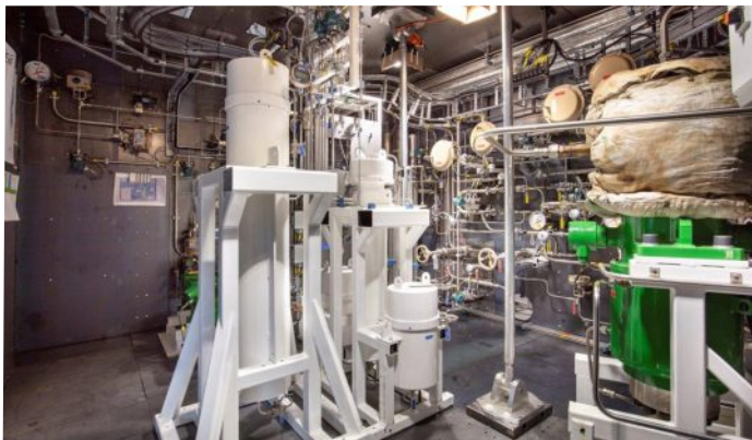
Overall view (purification filters in white)
