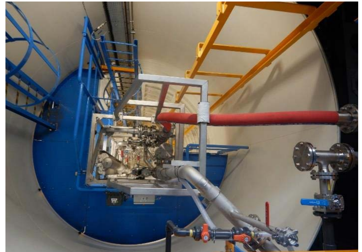
CORALIE Loop at the TOTEM facility (2022)
