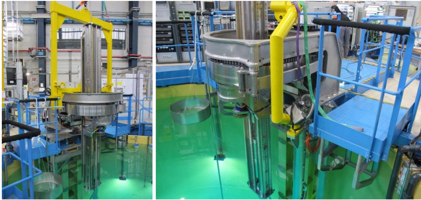
Installation of bench B installation in the CESARINE pool of the TOTEM facility
