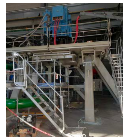
Primary circuit pump
