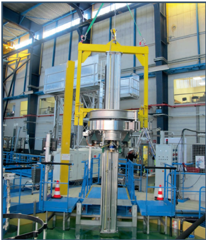
Disassembly of the UGXR bench in preparation for its return to the manufacturer (IDOM) workshop
