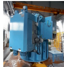
Primary pump motor
