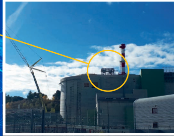
Lifting of modules onto the roof of BUA using a 450-ton crane
