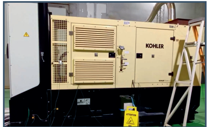
Thermal testing of the emergency diesel generator
